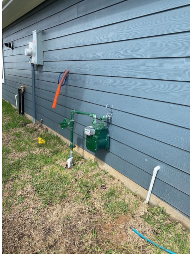
Type of Gas Distribution Piping Material: Cast Iron Comments:
